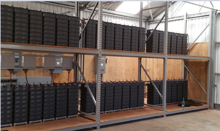
Forty Aquion battery stacks are used to power a 25-kilowatt installation at Mari's Garden, a nursery in Millani, Hawaii. The business's heavy power demand – combined with high Hawaiian electricity costs – made combining a solar PV array with Aquion batteries a smart financial decision. (Photo courtesy of Aquion)
