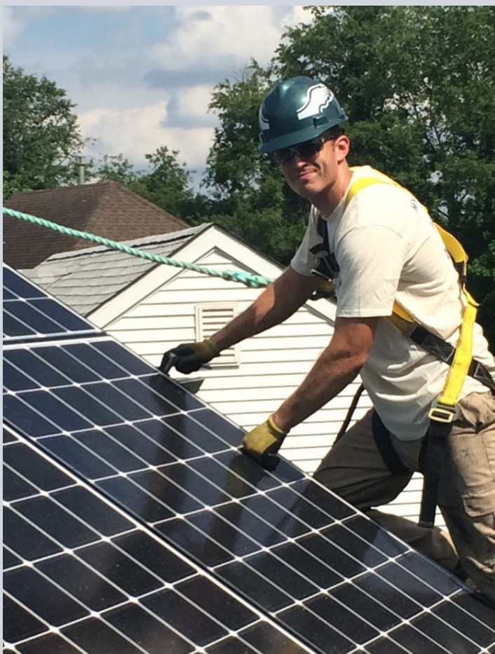
Michael Skala of Yardley, Pa.-based Exact Solar installs a solar array on a residential rooftop. (Photo courtesy of Exact Solar)
