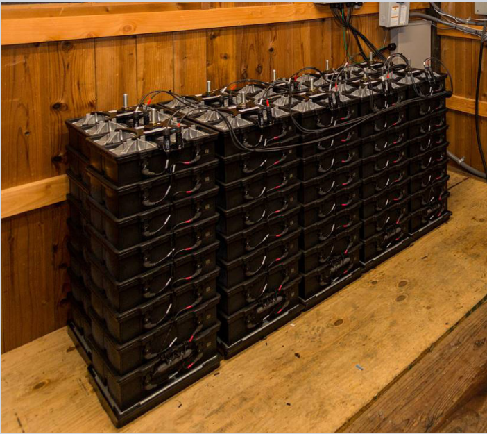
Aquion's batteries help solar energy power the operations at an off-the-grid ranch in California. Used worldwide, Aquion's batteries are produced in a large, high-tech manufacturing facility in Westmoreland County, Pa. (Photo courtesy of Aquion Energy)
