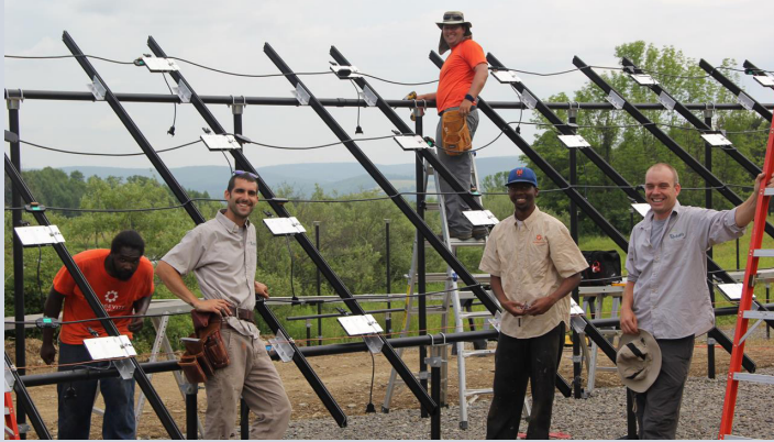
Taitem Engineering workers help install a solar array. Based in Ithaca, Taitem now has more than 45 employees. (Photo courtesy of Taitem)
