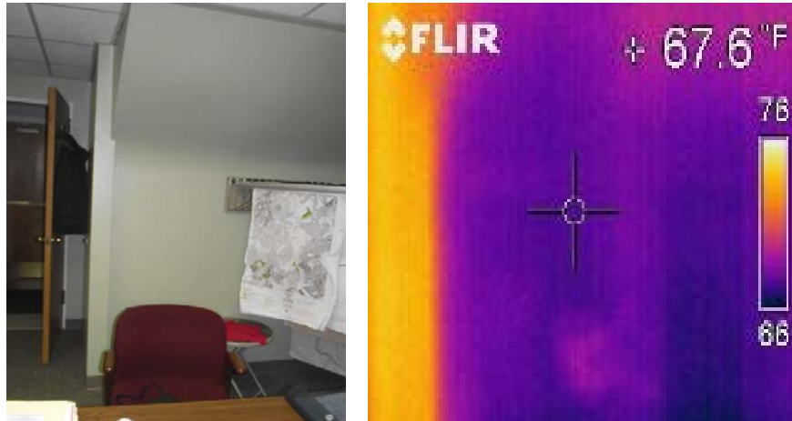
Figure 7: Air infiltration shown with infrared camera (right image)
