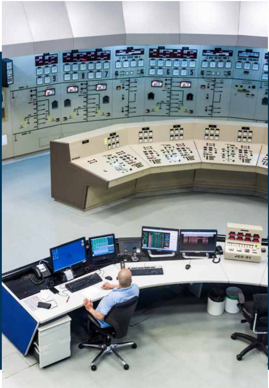
Command room of Itaipu dam on Parana River on the border of Brazil and Paraguay Photo: © Matyas Rehak/Shutterstock.com
