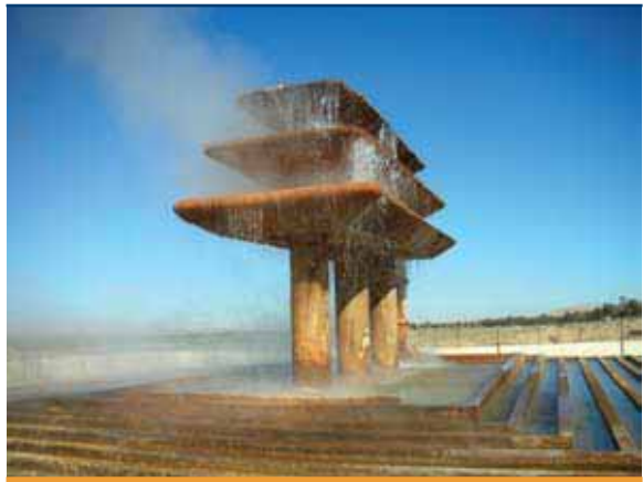
Figure 9.1 Cooling Tower Bringing Geothermal Water from the Sahara Down to a Temperature Usable in Irrigation
