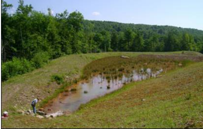
Passive Wetland Treatment System: Lausanne Tunnel water flows through pipes (forefront) into Wetland A (Photo: Wildlands Conservancy)
