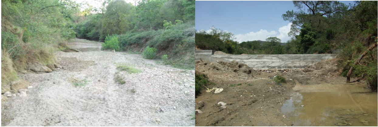
Check dam (before and after construction) at Tappa village in Himachal Pradesh
