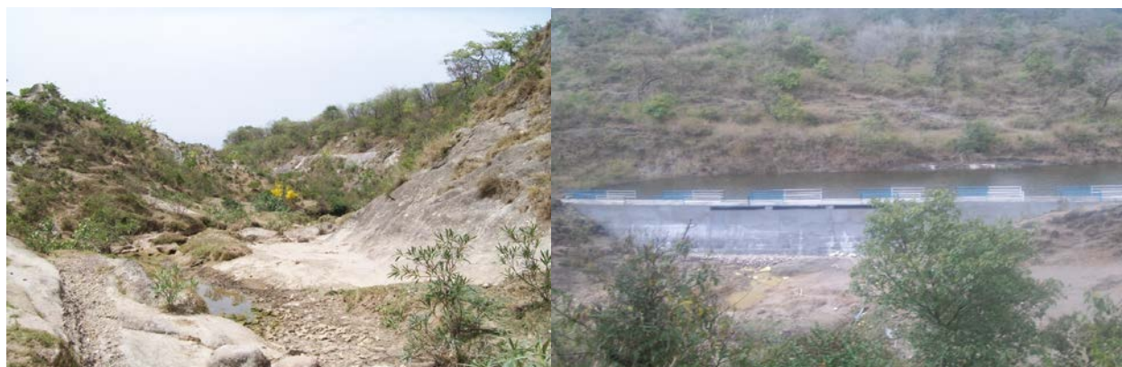
Check dam (before and after construction) at Nagrota Surin village in Himachal Pradesh
