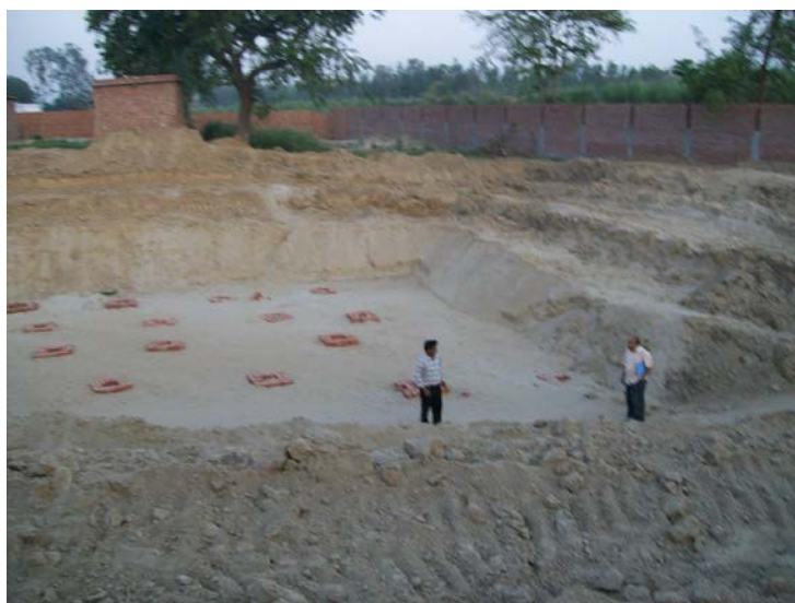
Figure 1. Farm pond showing recharge shafts on the bottom surface
