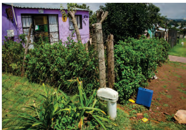
FIGURE 6: PREPAID METERS IN KAGISO, MOGALE CITY, SOUTH AFRICA
