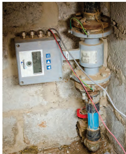
FIGURE 5: PREPAID METER ON AN INSTITUTIONAL CUSTOMER’S CONNECTION
