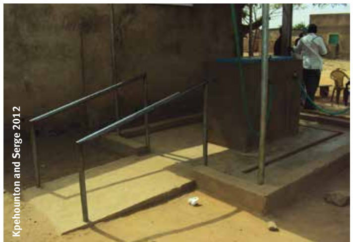
Figure 12: Waterpoint with ramp access and handrails, Burkina Faso.
