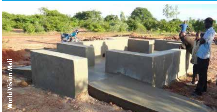
Figure 7: Accessible handpump apron, Moribila Zounoukan. Seating block is visible.
