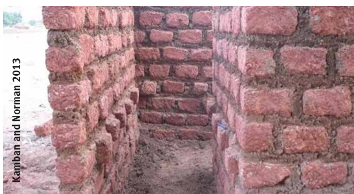
Figure 19: Latrine design with protruding bricks for support, and string for blind user to locate drop-hole.
