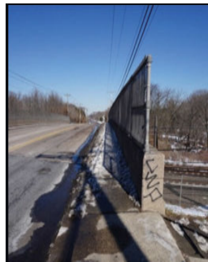
Snow-Covered Sidewalk on CR 673 Bridge (DVRPC, 2014)
