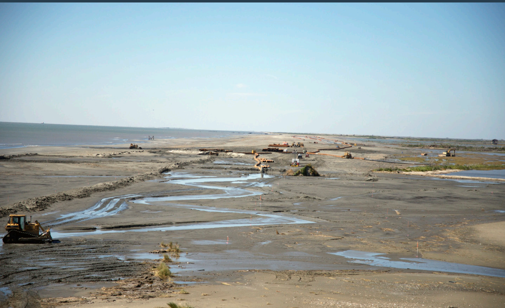
A hydraulic dredge pumps offshore sediment onto Chaland Island, an eroding barrier island in Plaquemines Parish. Source: NOAA
