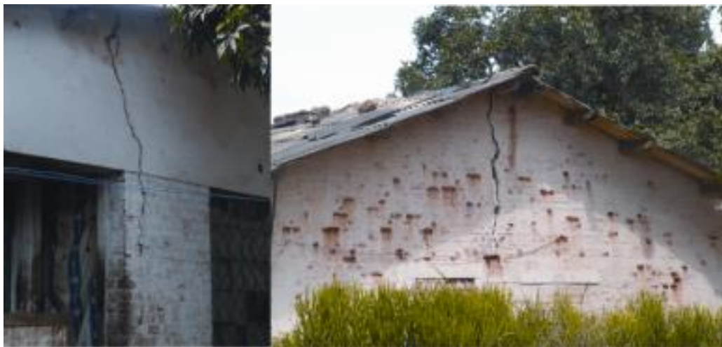
House in Musonoi. The cracks due to blasting of the mine T-17 are clear. Copyright: Bench Marks Foundation
