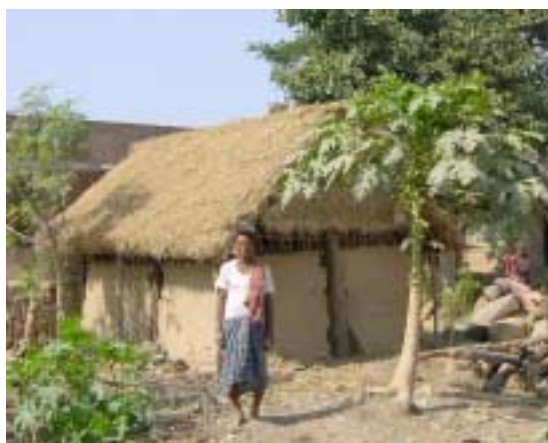
A new house under construction in Shrivantapur village, Jagatsingpur district, supported by VHAI and funded by DFID.
