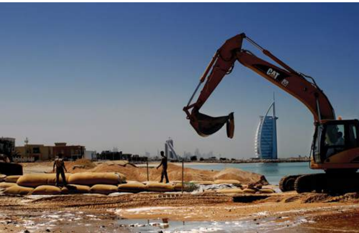
United Arab Emirates (UAE), Dubai. Migrant labourers working on extending the Dubai beach, close to the Burj Al Arab Hotel (right). The employers keep their employees' passports when they arrive and pay their workers around US$167 a month.
