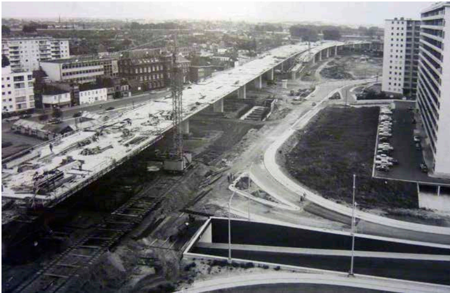
Figure 80 Construction of B401 viaduct in Ledeborg (Source: City Archives Ghent “Zwarte Doos”, GAGB series, nr. 462) (in: Druwé & Lalush, 2011)
