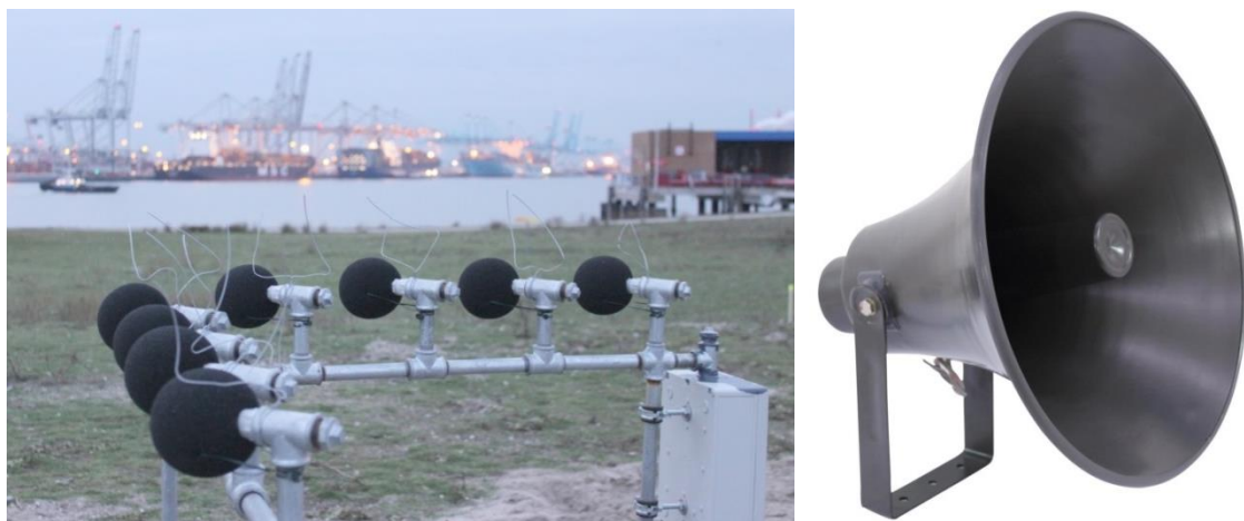
Figure 3: Example of an installed subarray with 8 microphones (left) and an Omnitronic NOH-40R loudspeaker, installed near the ground surface for audio synchronization (right).
