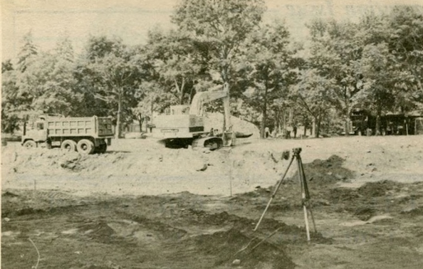
Construction of two new resident facilities on the corner of Husley and Eaton Street is currently underway over the summer to alleviate the housing problem on campus. Photo by Joseph E. Gaines
