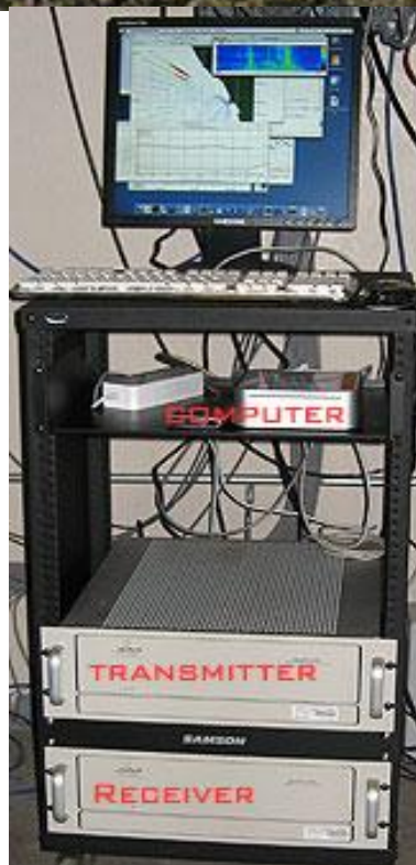
Figure 2.31 CODAR installation in California (UC Davis Bodega Laboratory)
