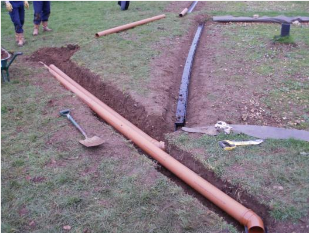
Figure 4-24 Tailwater runoff pipework
