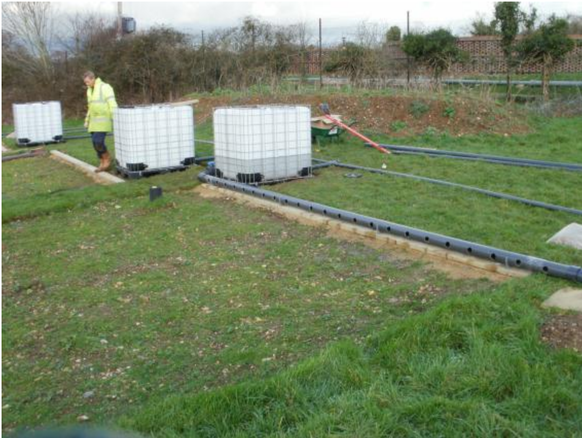
Figure 4-23 Irrigation tank and distribution chamber
