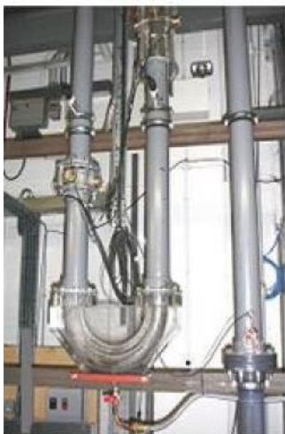
(b) Bottom section showing return BEND2, viewing section, and instrumentation
