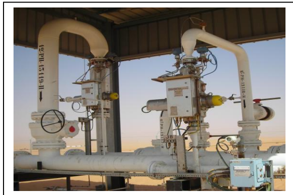
Figure A- 9, ROXAR MPFM installed in the El-Sharara oil field in Libya.
