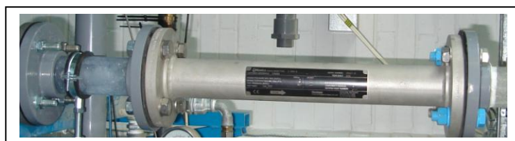
Figure 5-3, The Kenics static mixer installed downstream of Y-junction
