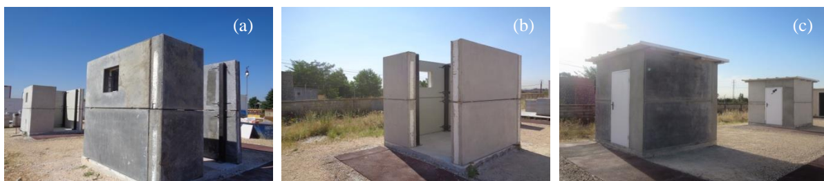
Figure 5 (a) SUS-CON panels mock-up, (b) reference panels mock-up, (c) two panels mock-ups finalized (front in the picture: SUS-CON; on the back: reference)
