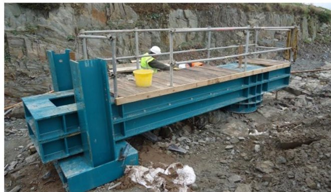
Figure 3 – Experimental apparatus. a) sketch of the shear testing rig when installed on site, representing also the applied loads and the adopted spatial reference system. f_h and f_v identify shear and normal forces, respectively. Superscript ^+ and ^- indicate the sign (positive or negative) of the applied loads according to the adopted sign convention. b) picture of the test rig system.
