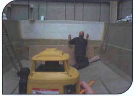
Using a rotary laser-level to mark the inside of the hull mould: providing a vertical reference datum to measure against.
