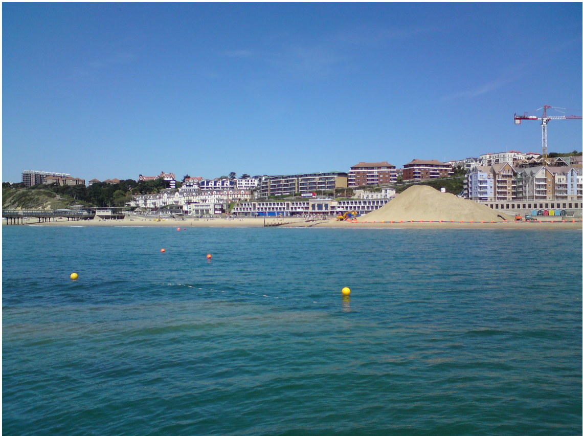
Figure (5.28). Photograph showing the sand pile during the construction phase, this sand is used to fill Boscombe ASR geotextile containers.
