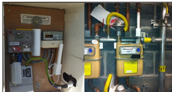
Figure 4 Pulse output sensors connected to the electricity meter (left) and gas meter (right)
