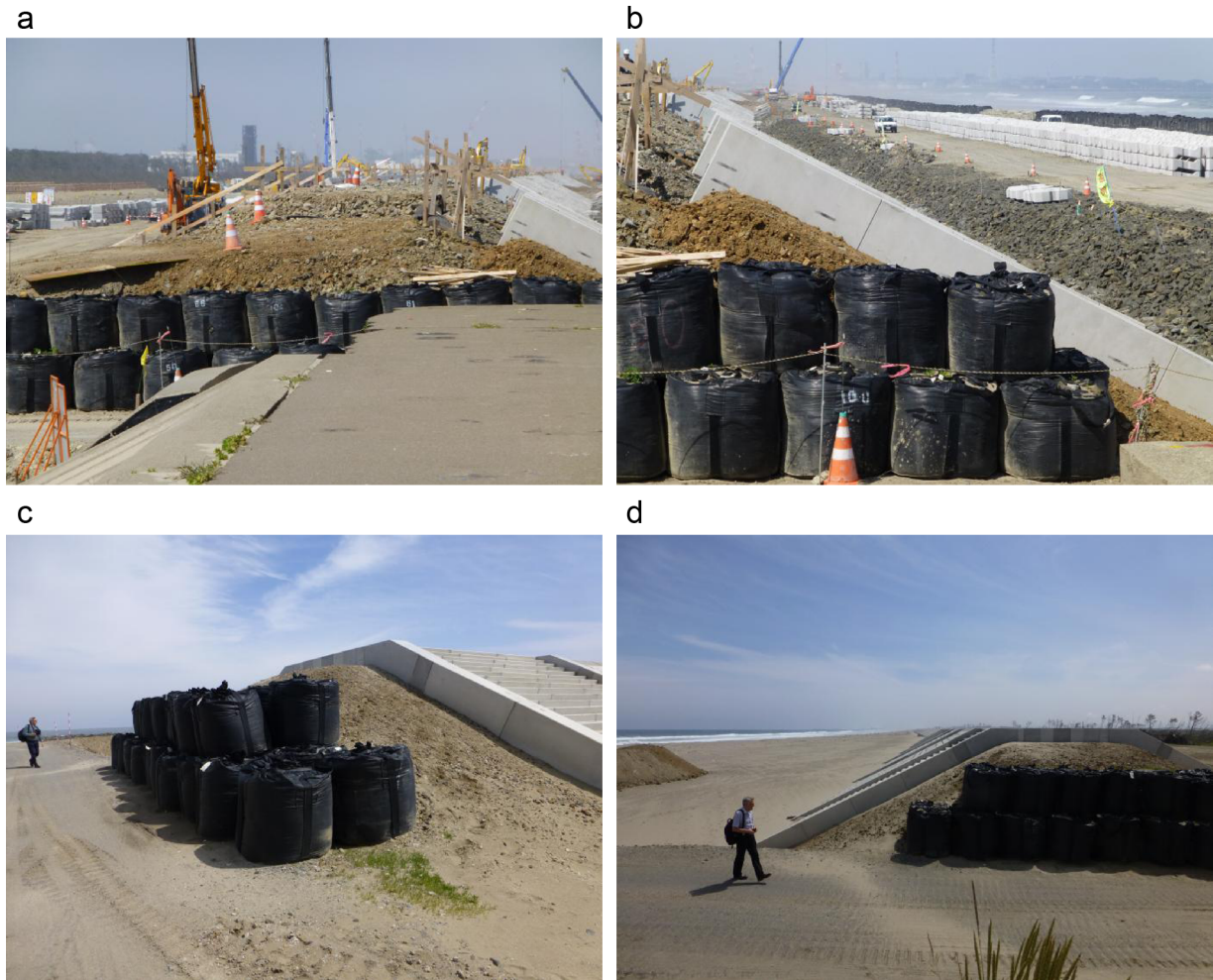
Fig. 14. Arahama sea dikes: (a) new portion under construction; (b) offshore side showing extent of construction site; (c) end of newly-completed portion south of the construction site; (d) looking southwards along completed portion.
