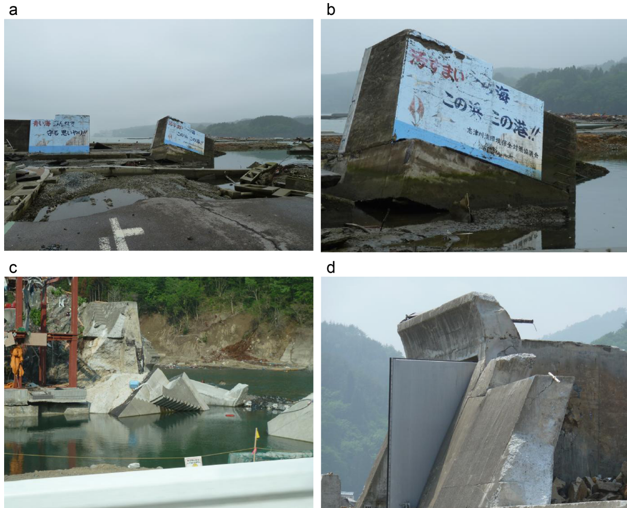
Fig. 8. Seawall damage observed during the 2011 EEFIT Mission: (a) damage to seawall and quay at Minamisanriku; (b) close-up of seawall block at Minamisanriku showing no interlinkages; (c) recovery work on the seawall at Miyako Bay; and (d) remaining seawall buttress at Tarō.
