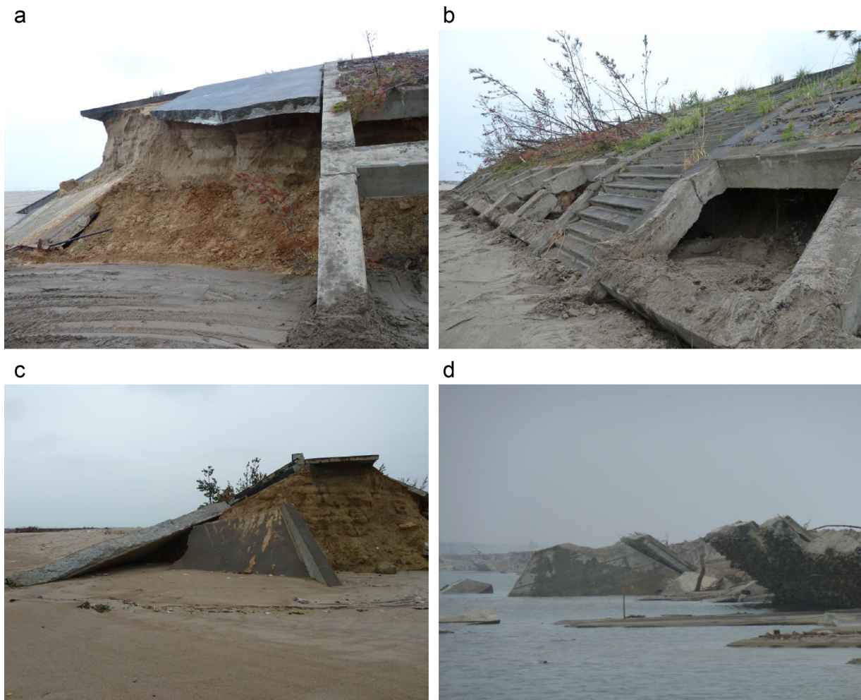
Fig. 7. Damage to Yamamoto sea dikes observed during the 2011 EEFIT mission: (a) exposed sand core on the lee side; (b) evidence of sand core having been washed out; (c) exposed section through the sea dike; and (d) remnants of the dike into the distance, lying in pools of seawater to the lee side of the structure having not subsequently drained away.
