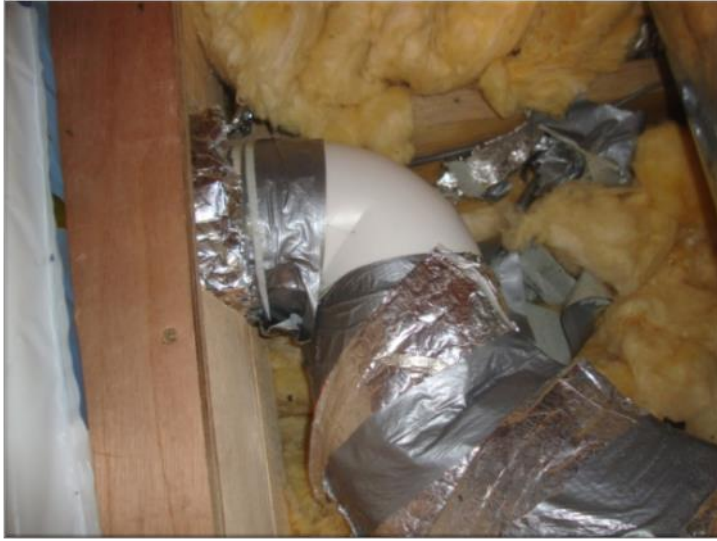
Figure 5. Duct bend un-insulated in cold roof (Source: Eco-Energy NI)
