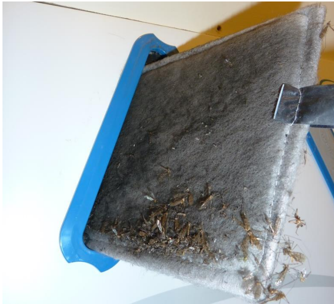
Figure 7. Inadequately maintained filters (Source: MEARU)
