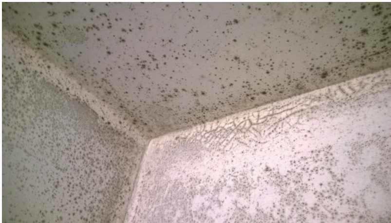
Figure 1. Mould growth on the ceiling of a poorly ventilated bathroom (Source: MEARU – Mackintosh Environmental Research Unit, Glasgow School of Art)
