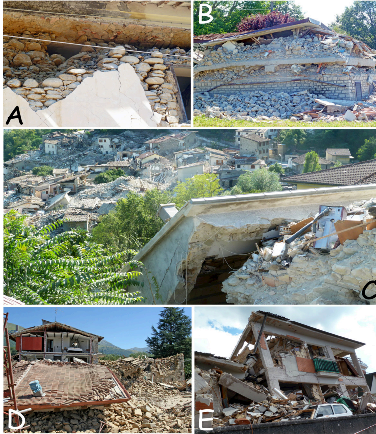
Figure 1. A, Rounded, fluvial cobbles masonry in Sommati (Amatrice). B, Collapse of a stone masonry building with RC ring beams (San Lorenzo e Flaviano, Amatrice). C, Crashed RC roof over a stone masonry house; in the background, view of the destroyed village of Pescara del Tronto (10-11 MCS). D, Collapse of stone masonry house in Petrana; behind, note the part of the same building added interiorly with a steel moment-resisting frame. E, Collapse of a RC building in Amatrice.
