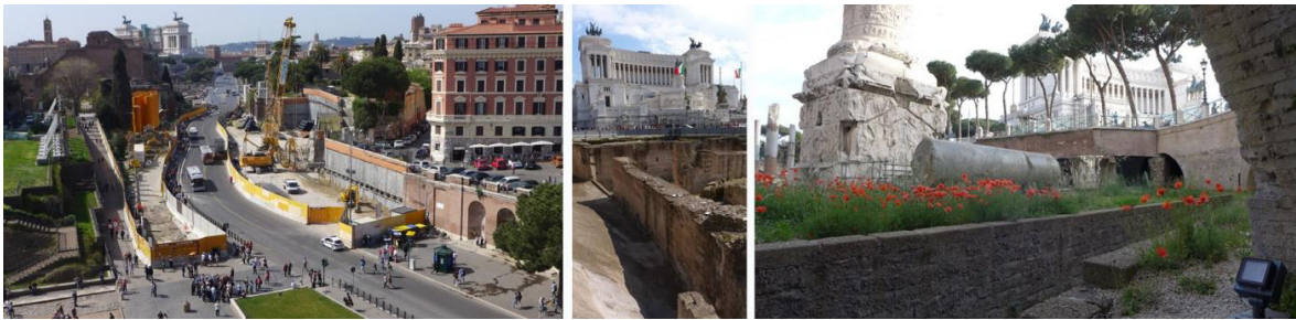
Fig. 8. Rome Metro Line C Left: Construction site at the foot of Colosseum and Basilica of Massenzio; the line runs just beneath Via dei Fori Imperiali, crossing all the area of the Imperial Fora. Center and Right: Archaeological level, including Trajan's Column, could be easily linked to transit spaces of the next station in Piazza Venezia.
