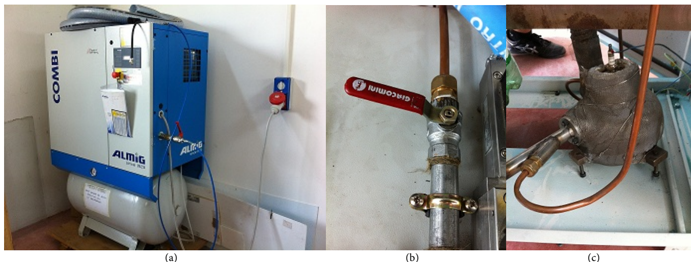
Figure 5. (a) Air supply; (b) the on-off manual valve; (c) copper air pipe into CC.
