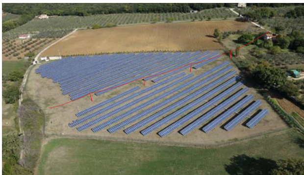
Fig. 1 PV plant in center of Italy crossed by a MV line
