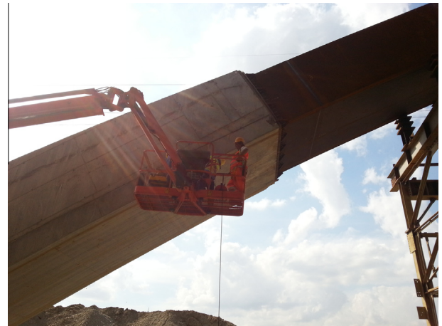
Fig. 2. Detail of the connection between the steel arch and supporting concrete flange.
