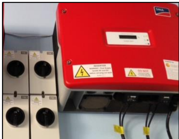
Figure 8.4: solar PV inverter and controls
