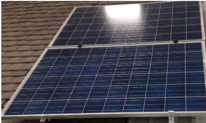
Figure 5.2: an example of the solar PV array installed within the school building
