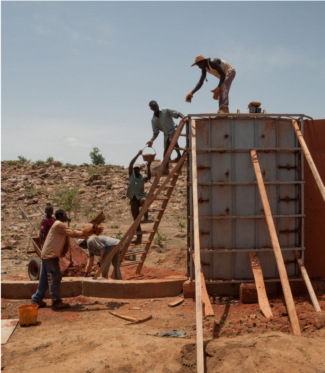
PICTURE 8. Secondary School project by Kéré Architecture and the community of Gando, Burkina Faso. Author: Emmanuel Dorsaz
