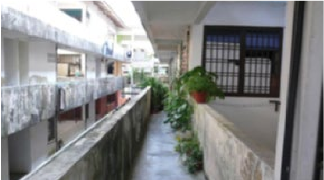
FIGURE 6. Planting along the small and narrow corridor becoming an obstruction to the people who pass
