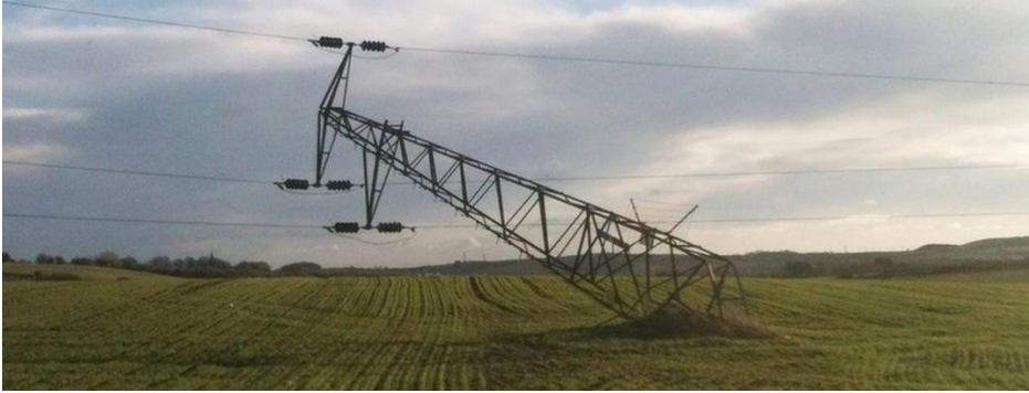
Figure 1: Damaged electricity pylon near Houghton-le-Spring, UK (BBC News, 2014)
