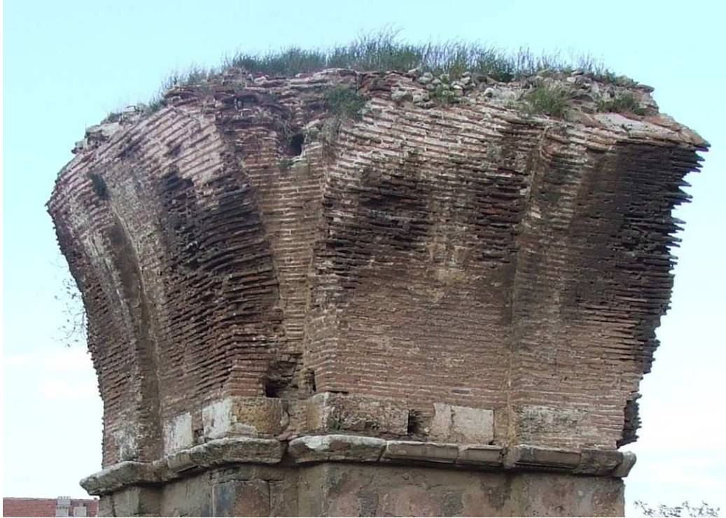
Fig. 10: Philadelphia, St. John, Detail of Vault Fragment on top of the Northeast Pier, displaying remains of a pendentive (photo by Nikolaos Karydis, 2007).
