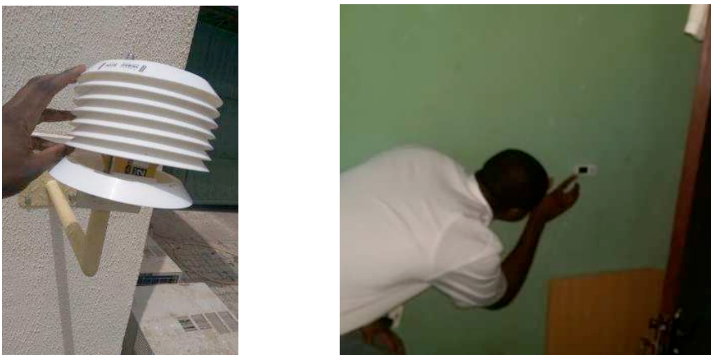
Figure 10: Installation of Tiny Tag outdoor logger and indoor Hobo T/RH sensors
