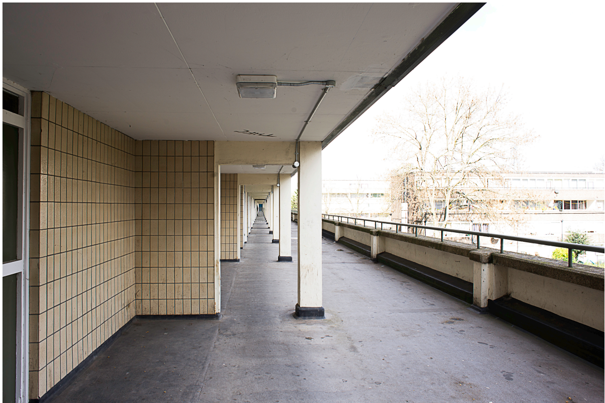
Figure 5 First floor walkway at Wendover. Some residents walk under the covered area in case material is thrown from high flats above (photo by author, 2014)
