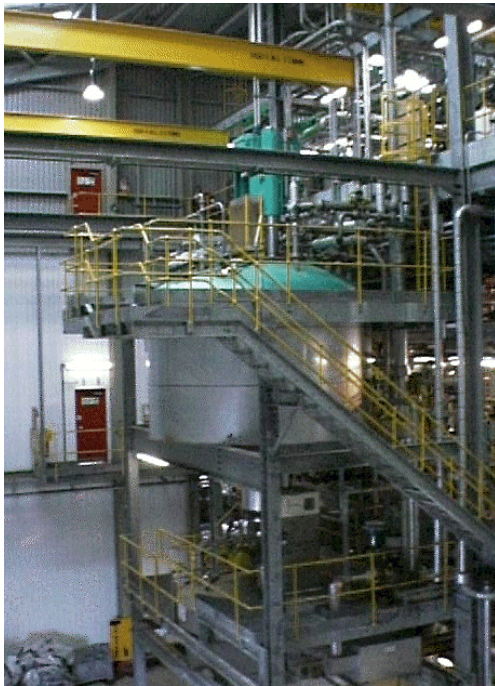
Figure 6.1: Side view of filter 24/970
