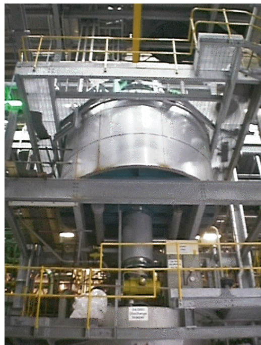
Figure 6.2: Underside view of filter 24/970
