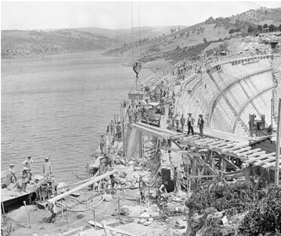
Figure 3. The Marathon dam under construction in 1928. ( Source: Photographic archive, Water Supply and Sewerage Corporation of Athens 1995).
