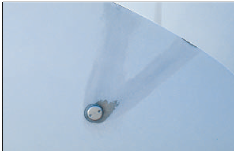
Figure 3 Tip of blade with surface erosion caused by lightning arc around receptor and towards the trailing edge [32]
