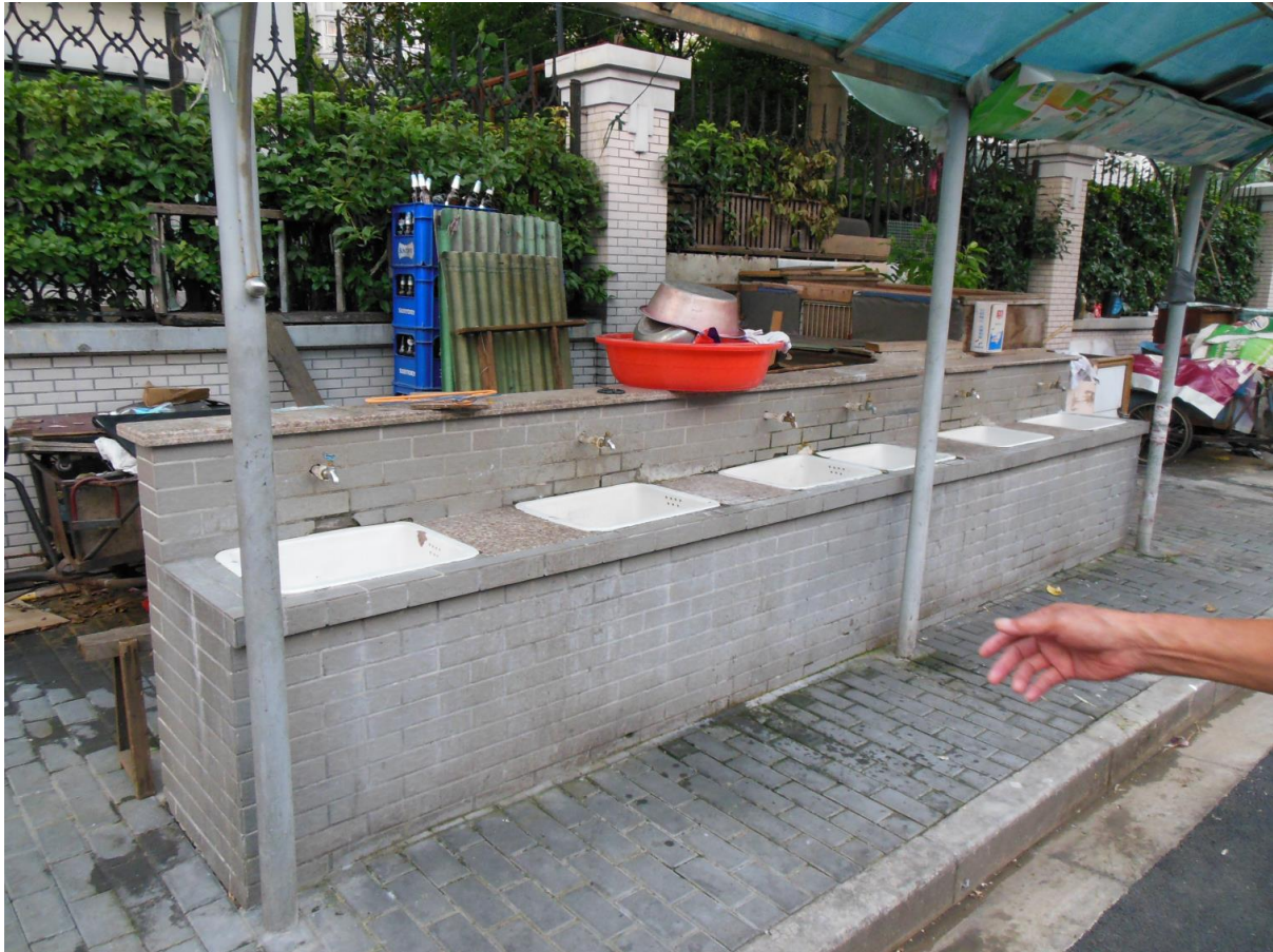
Figure 3: Public water taps, built for local residents in expectation of the EXPO 2010. Photo: the author, 2013.
