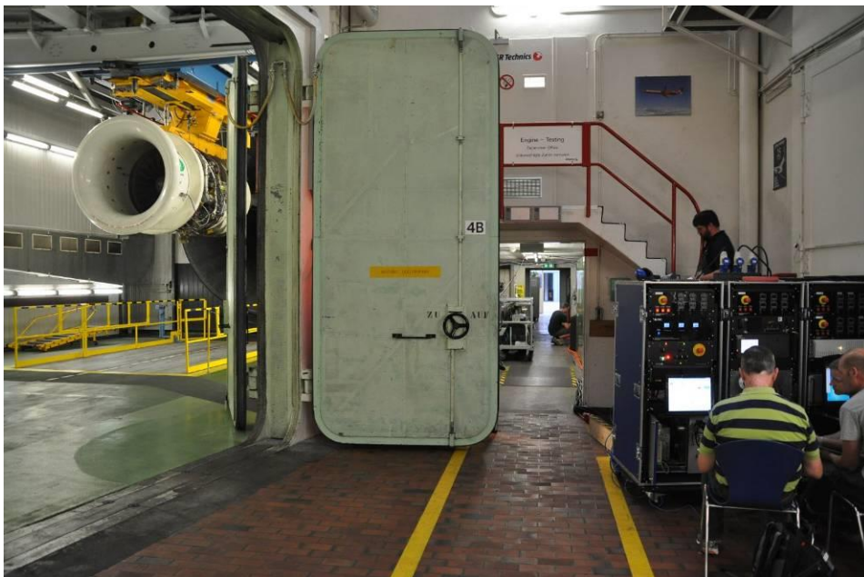
Figure 38 Photograph of EU/EASA Mobile Reference System location next to SR Technics Test Cell
