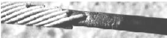
Fig. 2. Damage on a polyethylene sheathed cable on 100 kV line in Chile. The metallic wires on the left are part of the cable clamping system at the tower.
