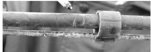
Fig. 14. Damage on the cable and rod can be seen. The clip used here is for a larger sized cable, and is too loose on the ADSS cable.
