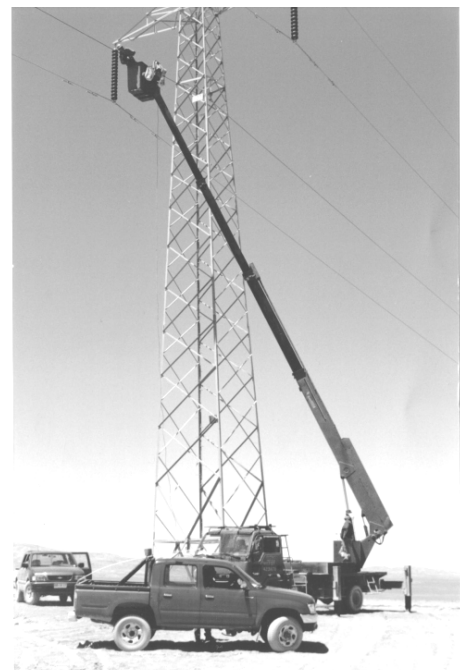
Fig. 11. An installation in Chile using a cherry-picker. This approach was used on all lattice towers.
