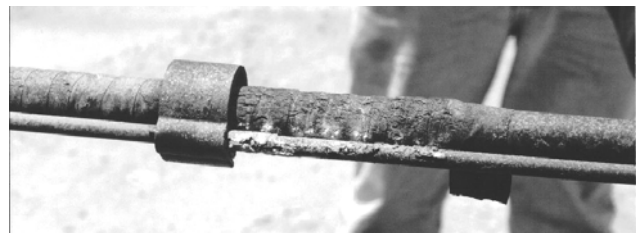
Fig. 15. Damage to the rod which is running over a wrapped semiconductive repair sleeve.
