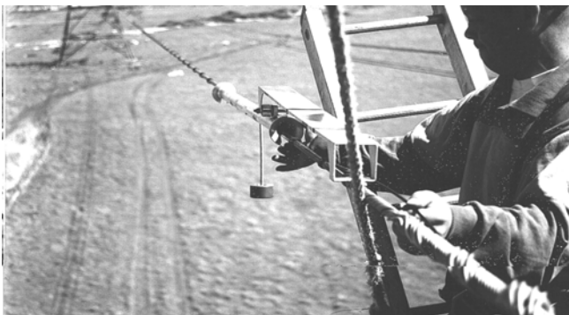
Fig. 10. An installation on a 400 kV tower in the UK. The linesman's right hand is touching the split-tube running earth, his left hand is pushing the rod into the span; he attaches clips between these positions.
