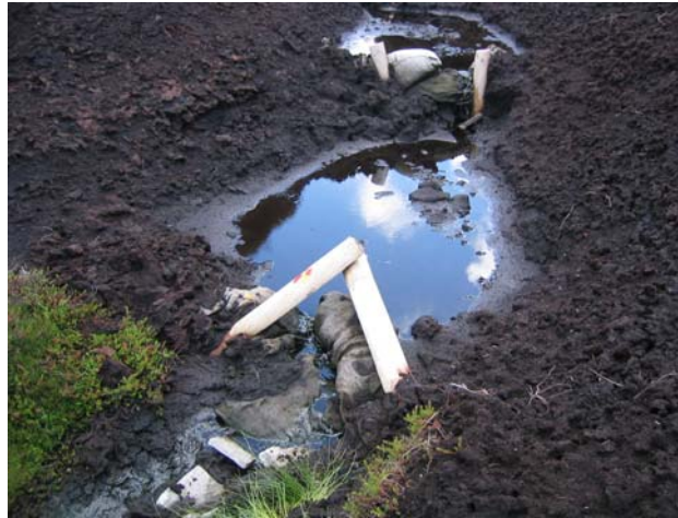
Figure 2.6 Wool bags anchored with wooden stakes. The majority of these dams are positioned in downstream locations where gullies are deep and wide bottomed.
