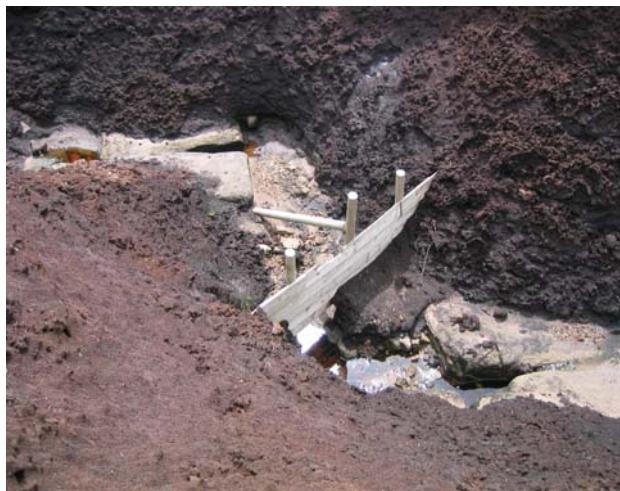
Figure 2.13 Undercutting by water of a wooden gully block. Any sediment trapped behind dam has been washed away underneath dam.
