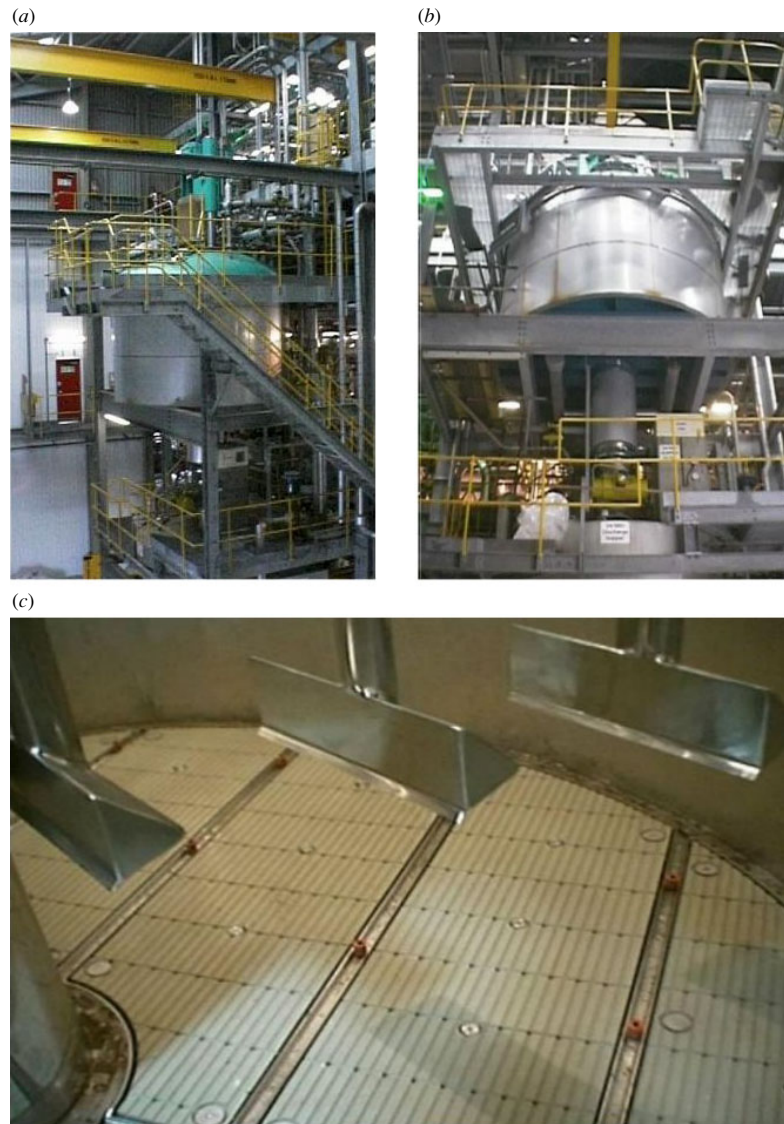
Figure 1. Views of the 36 m 3 ProceMon pressure filter; (a) and (b) external views and (c) internal view showing agitator blades and fixing bases for supporting the filter cloth.
