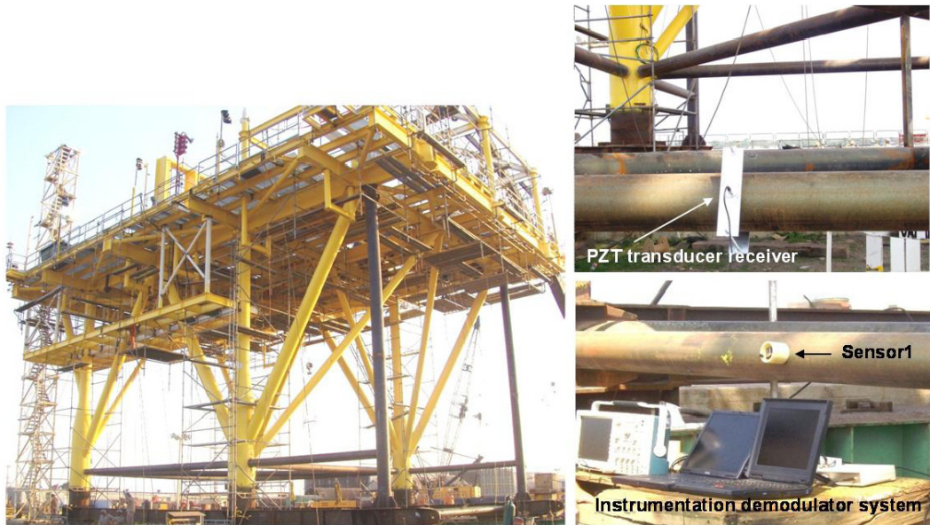
Figure 13. Experiment setup using the base deck of an oilrig under construction, its sensor modulator, its PZT transducer receiver and the instrumentation demodulator system.
