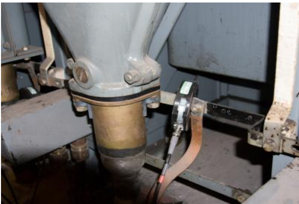
Figure 2 High frequency current transformer sensor attachment
