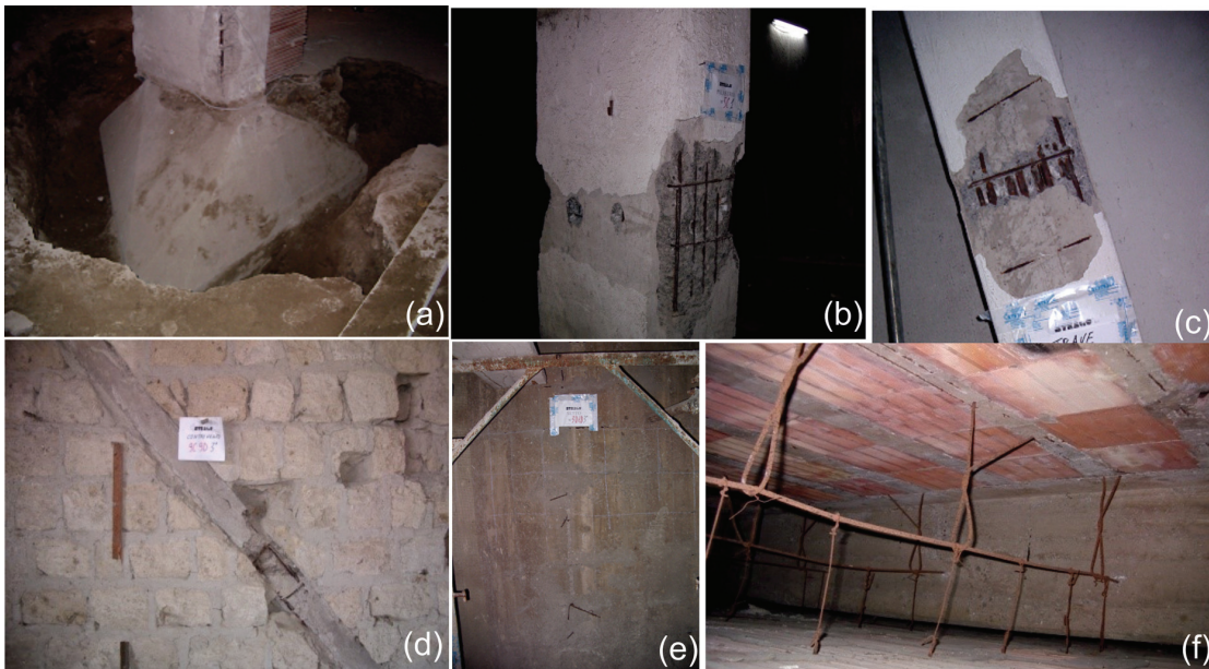
Figure 4. In situ inspections: (a) foundation footing; (b) columns' and (c) beams' reinforcement; (d) concrete diagonal brace in tuff masonry infill; (e) concrete infill; (f) floor slabs (De Luca et al., 2014)
