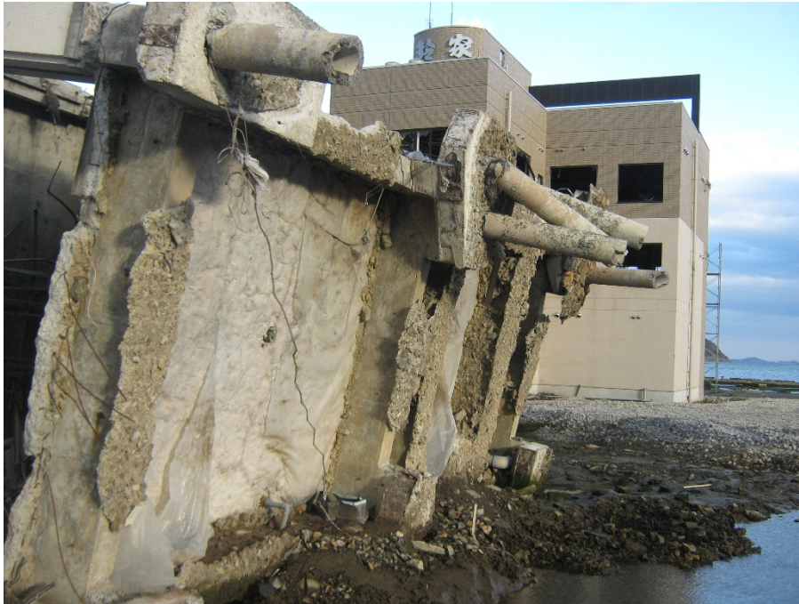
Figure 3: Collapse of a pile-supported building in Onagawa
